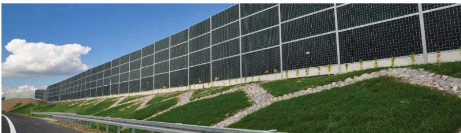
Figure 10E.6: Metal / composite noise barrier, on top of a bund
