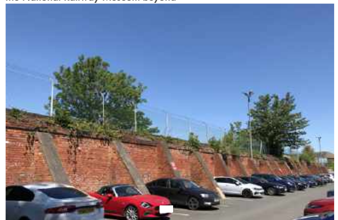
Fig.264 Coal drops with the original coal cells trimmed back to form buttresses
