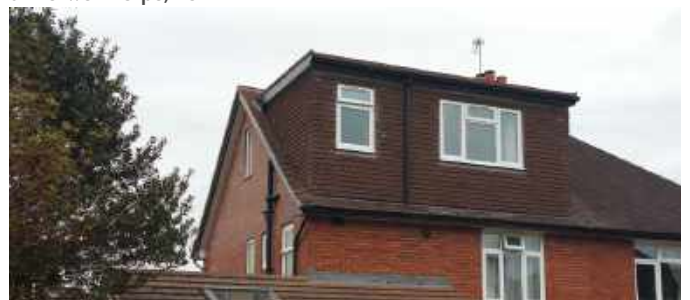
Fig.327 Not integrated with facade, dormer too big (dominates the roofline and elevation), windows too small, no articulation of dormer elevation, roof slope shows cheap roofing material, exposed gutter delivering to roof
