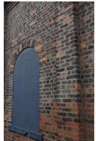
Fig.242 Cement pointing ideally should be replaced with lime-based mortar pointing
