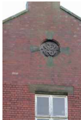
Fig.241 Inappropriate cement pointing
